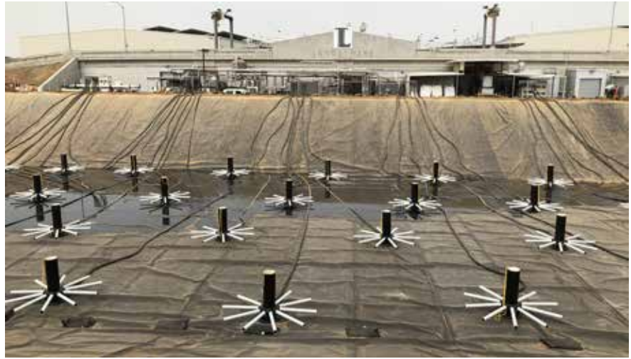
Instead of traditional floating aerators, the Lange Twins deployed Ares aerators from Triplepoint Environmental that are placed on the bottom of the pond. The aerators disburse fine and coarse bubbles that add and mix throughout the pond.
