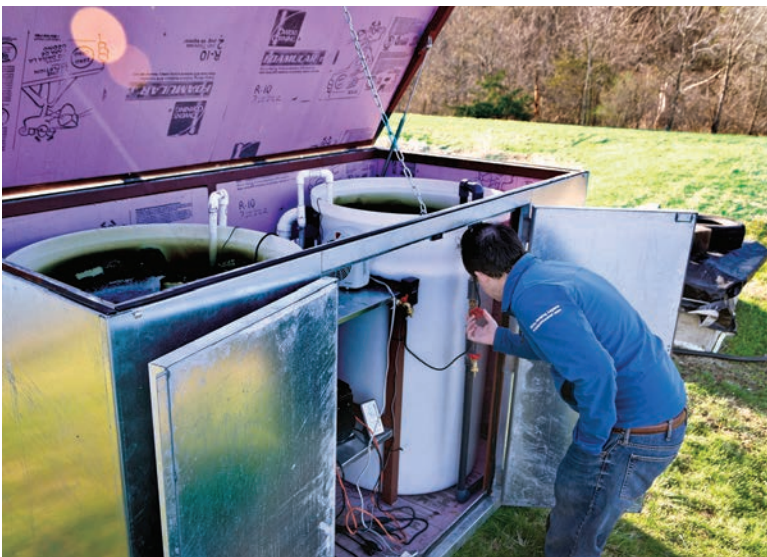
Brady O'Leary of Triplepoint prepared the NitrOx system for pilot testing.
