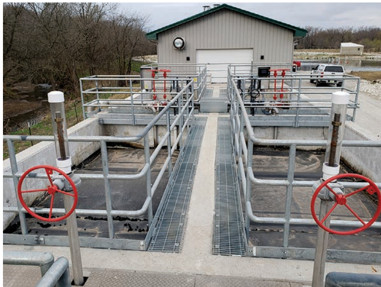
The four NitrOx cells are part of a $2 million facility upgrade in De Soto, Iowa.
